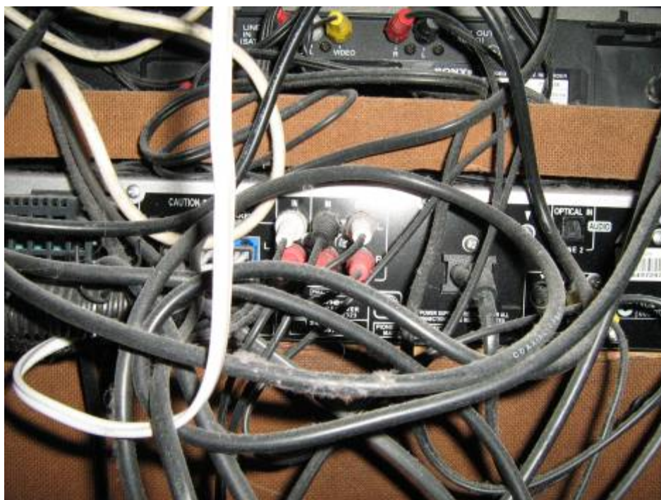
Figure 3: Complexity in cabling
