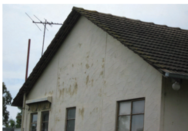
Example of weathered/poor condition of exterior wall and fittings.
