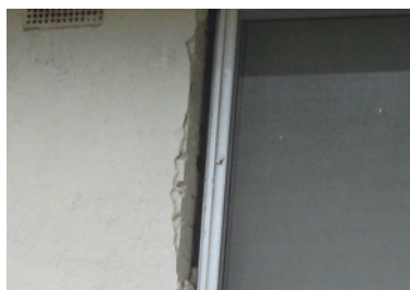
Example of reported gaps between wall and window, allowing ingress of weather.
