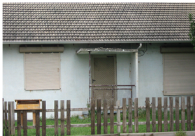
Example of poor condition of property.
