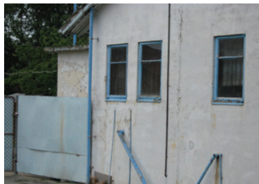
Example of poor condition of rear of dwelling.
