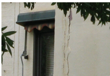
Example of cracks in exterior wall.
