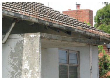
Deterioration of entrance-way and no maintenance of guttering.
