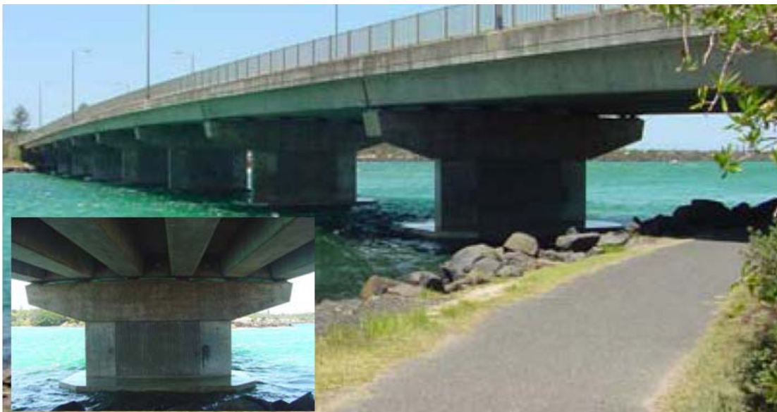
Figure 3-16 Bridge BD3 constructed in 1984 in the northern region of NSW (Source: RTA)
