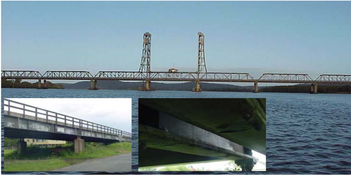
Figure 3-11 Bridge BD2 constructed in 1967 in the northern region of NSW (Source: RTA)
