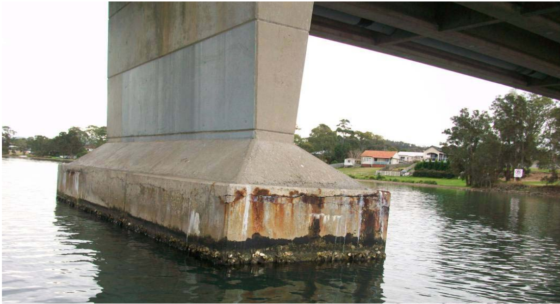
Deteriorated concrete columns of bridge structures (SOURCE: RTA)
