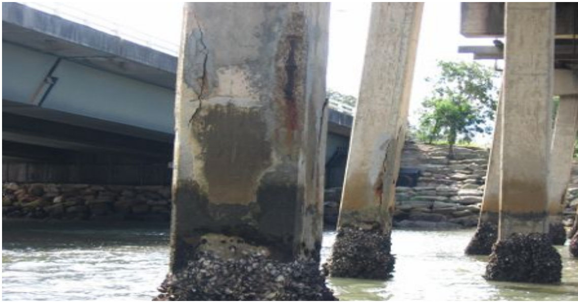
Cracked concrete bridge structures (SOURCE: RTA)
