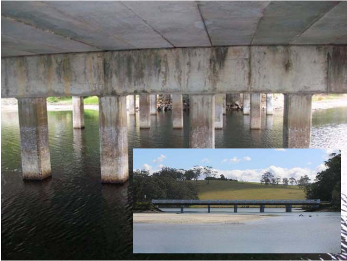
Figure 3-1 Bridge BA1 constructed in 1956 in the southern region of NSW (Source: RTA)
