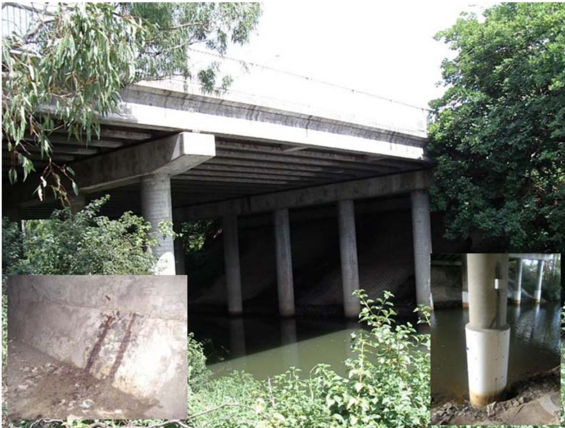
Figure 3-13 Bridge BA3 constructed in 1980, in the southern region of NSW (Source: RTA)
