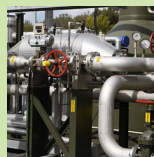
Bondi waste water treatment facility Location: Sydney Date of completion: 2009 Size: 2MW Source: Sydney Water
