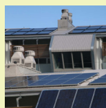
K2 Apartments, Melbourne Location: Melbourne, Vic Date of completion: 2008 Size: 21.4kWe Source: Arup project database
