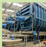
Eastern Creek UR3R Location: Sydney Date of completion: 2007 Size: 2MW Source: WSN
