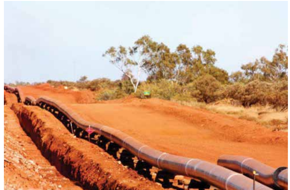
Gas pipeline construction corridor with welded steel pipeline and trench Photograph courtesy of Department of Mines and Petroleum
