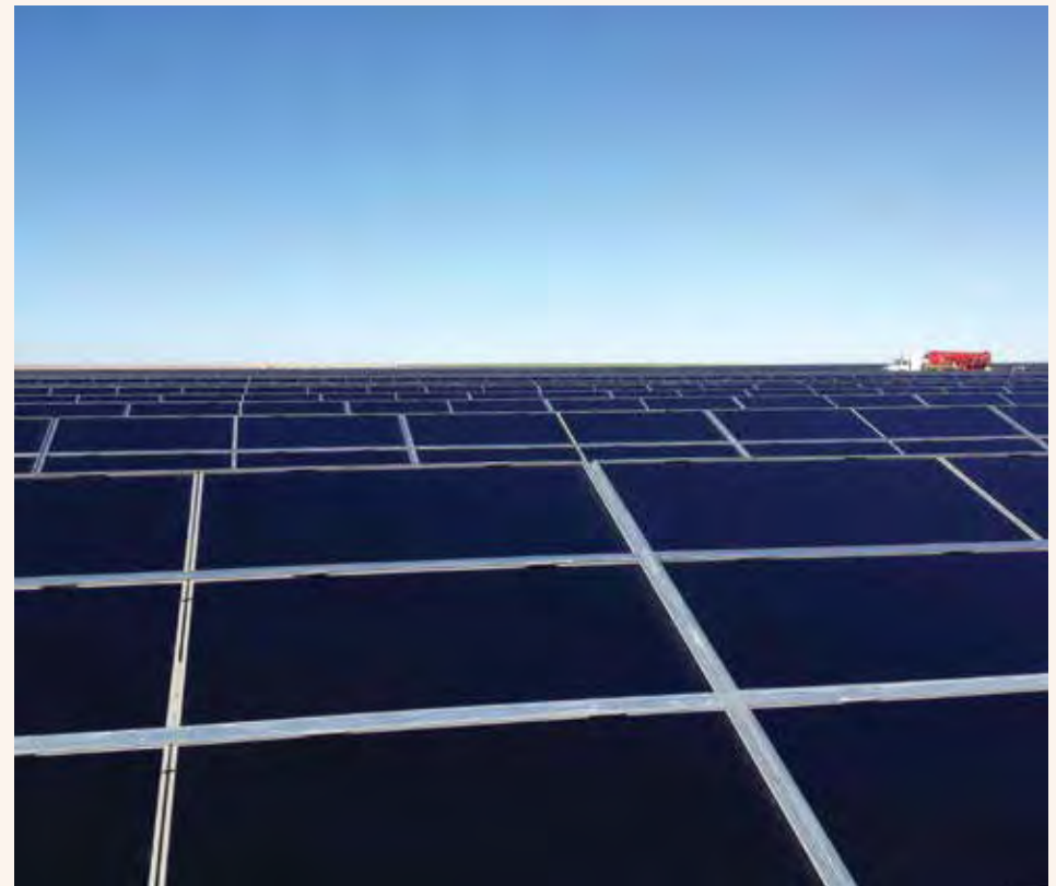
Solar Panels close up – Greenough River Solar Farm (Source DRD)
