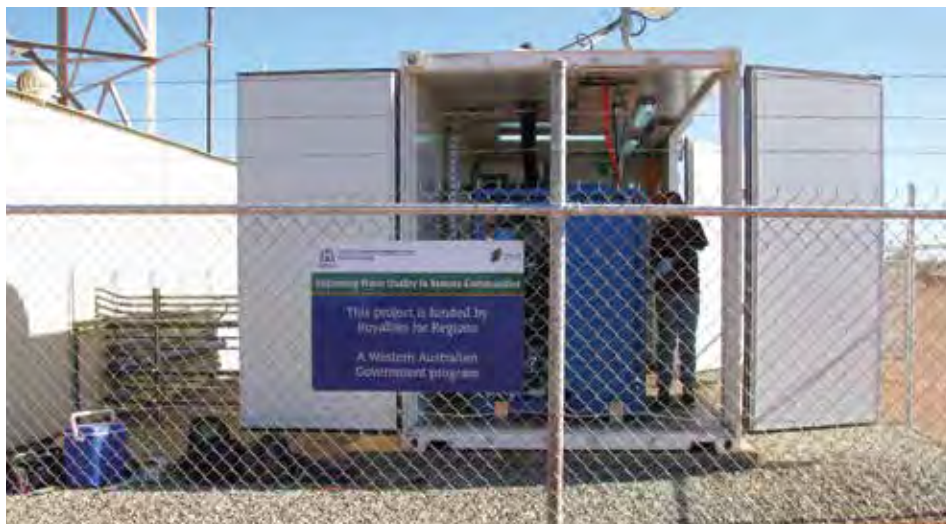
Installation of the Kiwirrikurra water treatment system (Source DRD)
