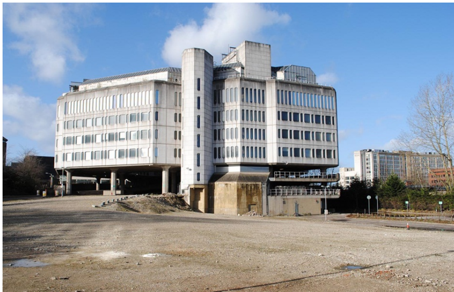
The Metal Box Head Office Building, Reading, following the demolition of low-rise staff facilities from the foreground.
