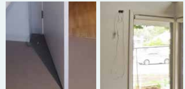
Slimline wall corner guards and timber-look vinyl flooring, Abbotsford (left) and pre-wiring for future blind automation prior to install of coverplates, TAC RIPL Housing (right).
