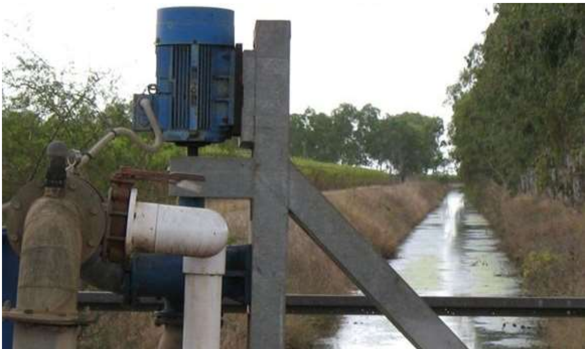
Figure 86. Pumping from a recycle pit – lower Burdekin
