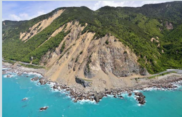
State highway and main trunk railway line buried by landslides at Ōhau point. Photo: Dougal Townsend
