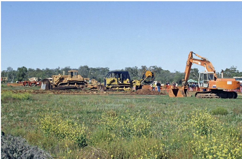
PIPE LAYING FIELD DAY, LIGHTNING RIDGE, NEW SOUTH WALES, 2001. PHOTO: G HOGAN
