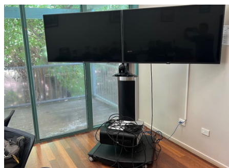
Figure 18: Videoconference facility in TSIRC Boardroom
