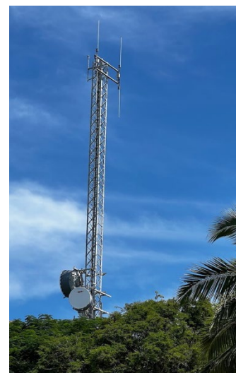
Figure 10: Telstra mobile tower in Medige Village
