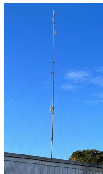
Figure 33: An Access Point had failed, limiting connectivity for a section of the community
