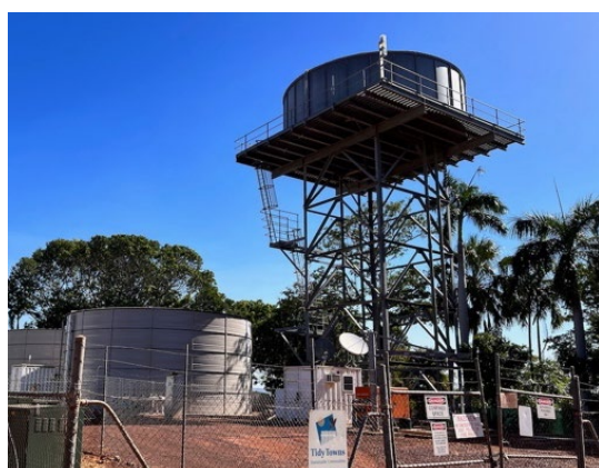
Figure 23: Telemetry is used to monitor the water treatment plant
