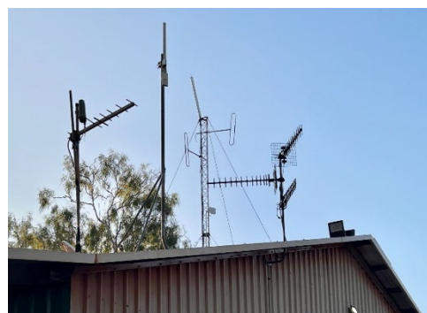
Figure 7: An array of communications equipment on the DAC office roof and broadcast tower
