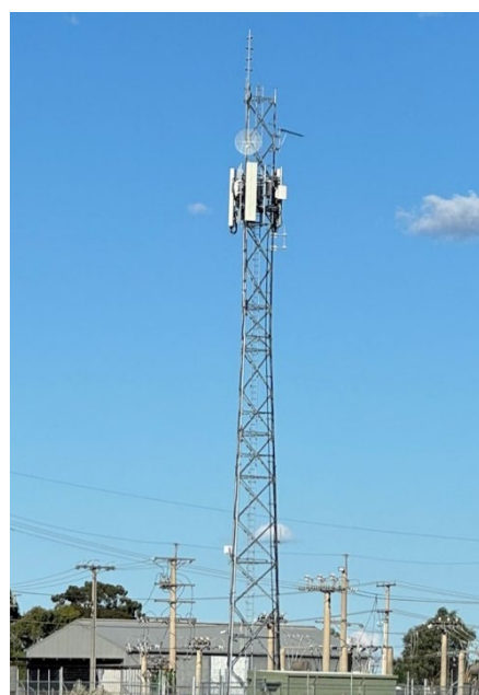
Figure 13: The new OneWiFi neutral host tower in Wilcannia
