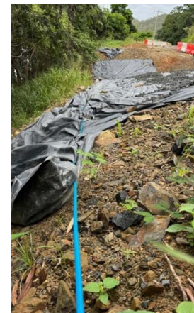
Figure 16: Replacement fibre optic cable at site of landslide
