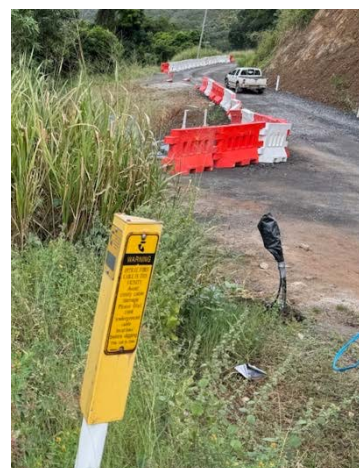
Figure 12: Road section where landslide occurred awaiting repair, May 2024
