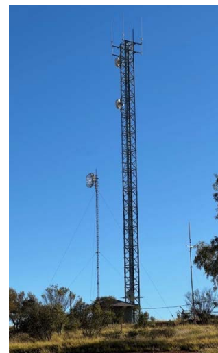
Figure 8: The new 40m 4G tower in Yuelamu was activated in June 2023. The other towers are the HCRC microwave link (left) and radio broadcasting (right)
