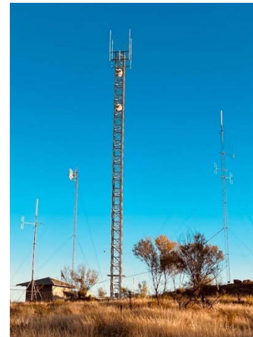
Figure 14: The 4G mobile tower awaited activation for 8 months
