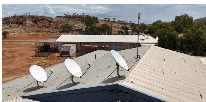
Figure 14: Three NBN satellite dishes on the PY Ku Centre provide backhaul for the Wi-Fi mesh network
