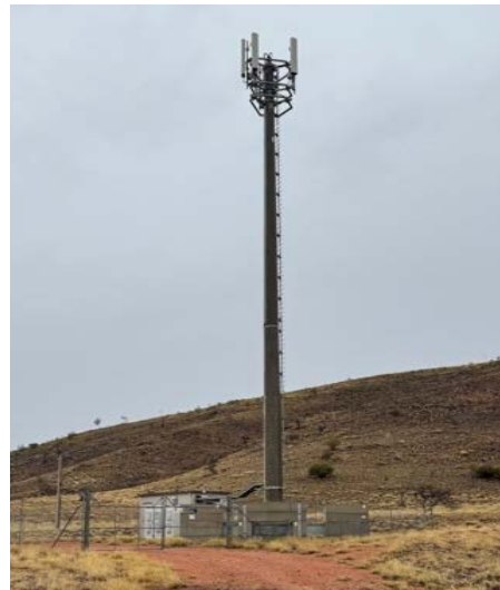
Figure 4: Pipalyatjara mobile tower
