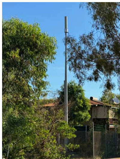
Djarindjin small cell mobile tower
