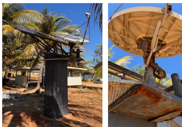
Figure 15: The Wi-Fi phone unit at Ngayawili homeland was quite rusty with the phone not working (2024)
