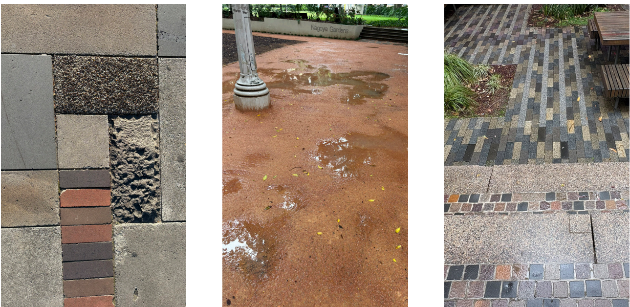
Figure 32: Inconsistent surfaces increase the chance of tripping over
