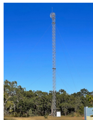
Figure 9: The HCRC tower for Telstra phone services
